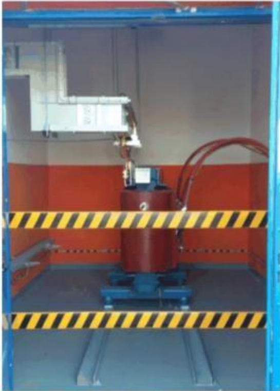
Photo. 11. Example of arrangement of protective barriers in the transformer chamber.
