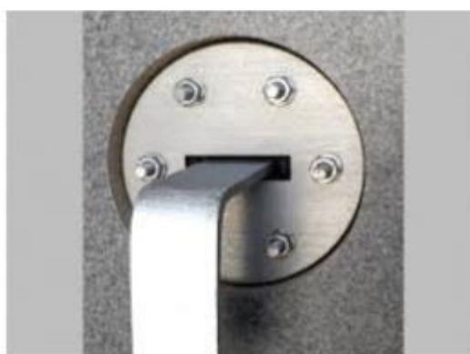
Photo. 9. Grommet for leading flat strip through a substation wall.
