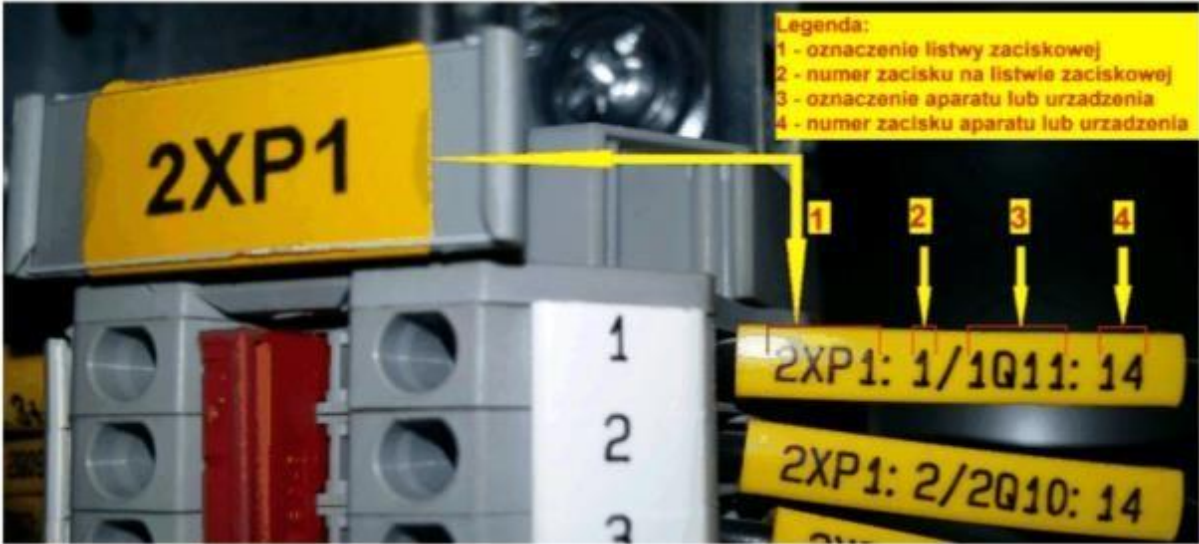
Photo. 7. Example of addressing wires on a marker
