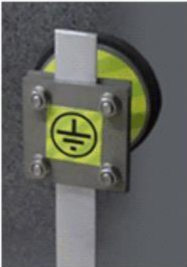
Photo. 13. Tight bolted grommet used for leading earthing flat strip
